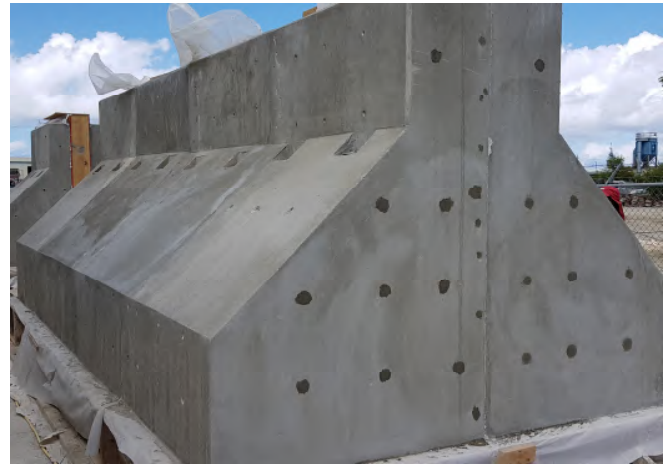
Concrete Modules for Mitigation Gate
